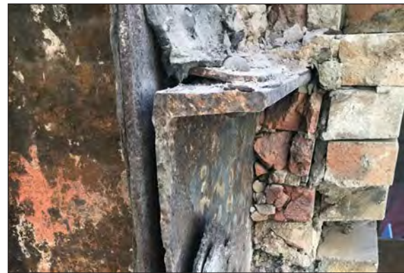
■ Engineering probe of the Community House Facade, showing the effects of steel expansion on a masonry wall.
