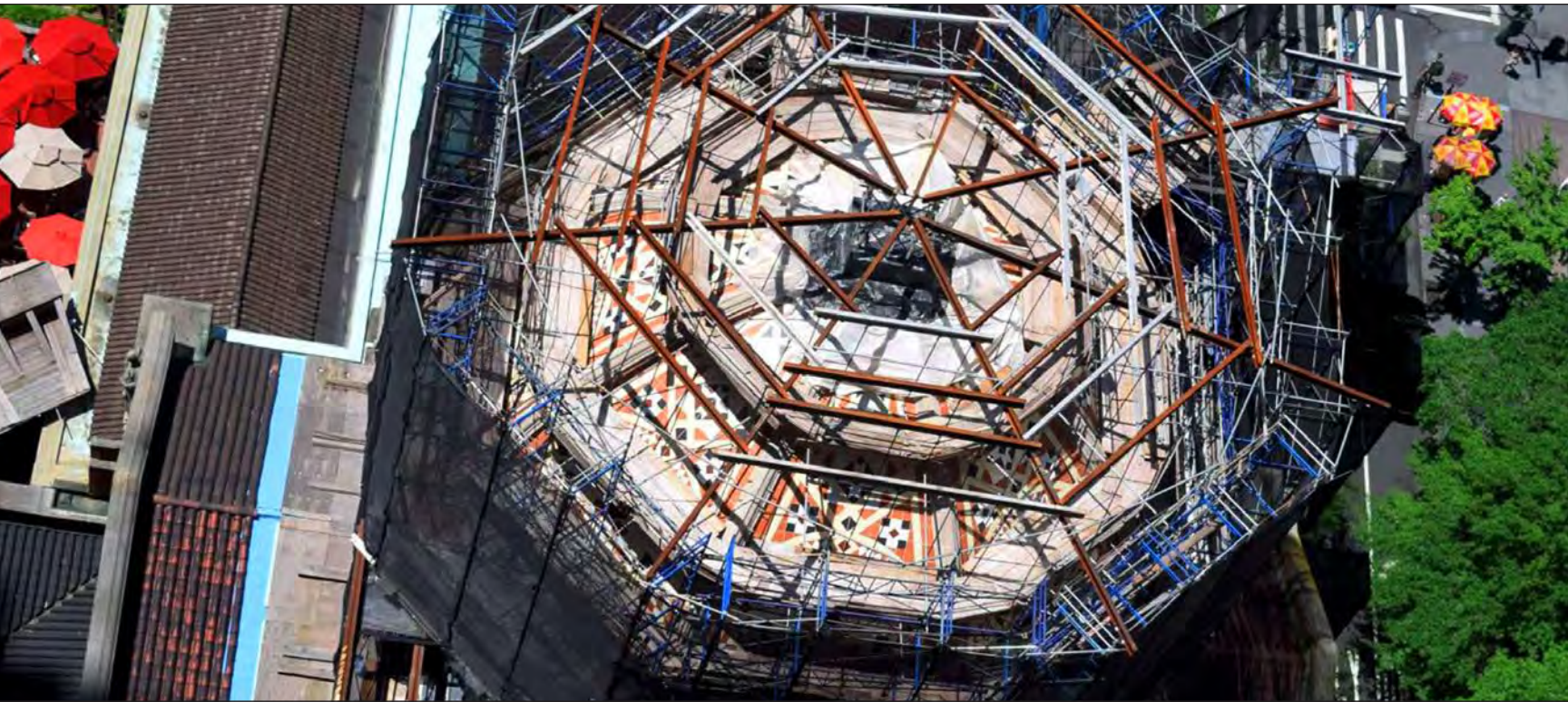
■ EarthCam, Inc. view of the Great Dome restoration atop St. Bartholomew's Church, July 2017.
