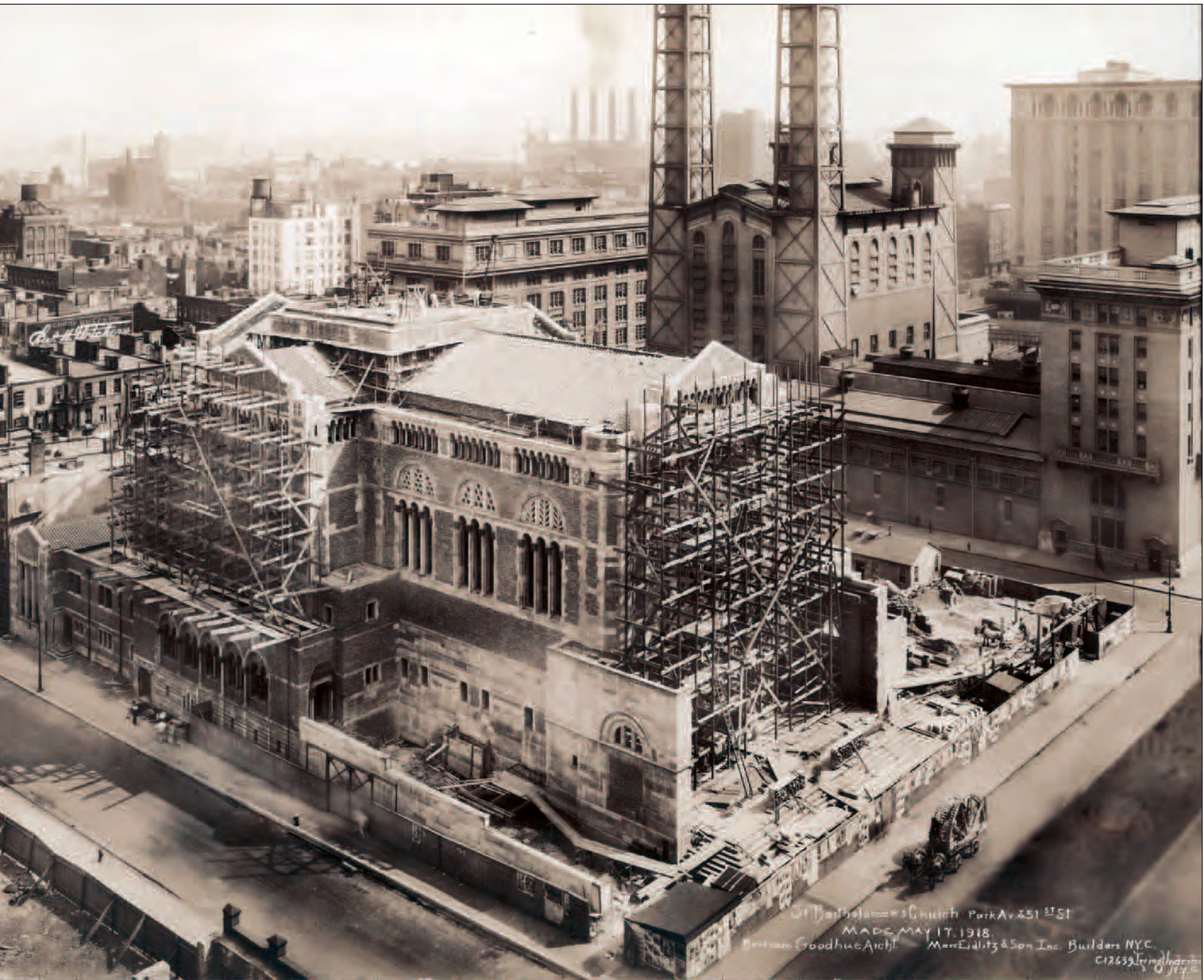
■ St. Bartholomew's Church undergoing construction on Park Avenue, May 17, 1918. Opposite: Construction workers and scaffolding atop the Dome, July 2016.
