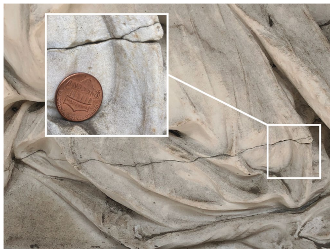
Large Lateral Crack Bottom Left, Central Tympanum.
