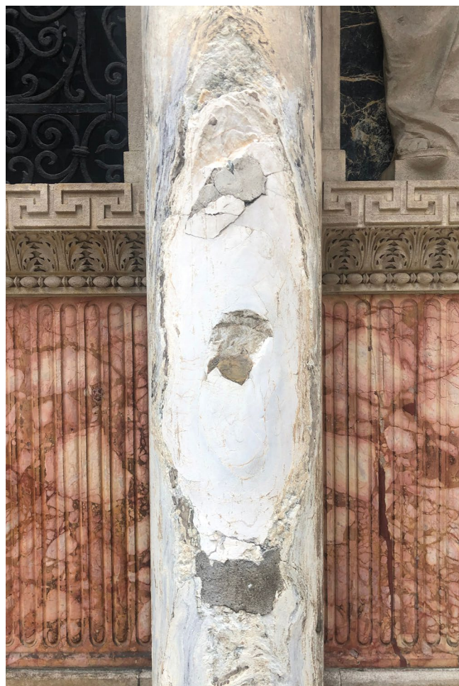
Detail: Incompatible/Mismatched Patches.
